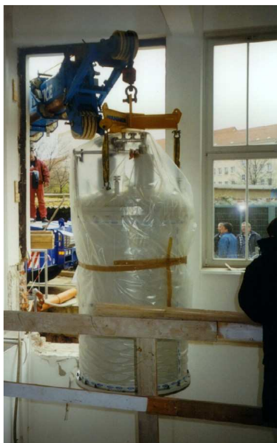
Figure 2: The magnet of the AVANCE 750 comes into our building through a big window (height approx. 4 m)
